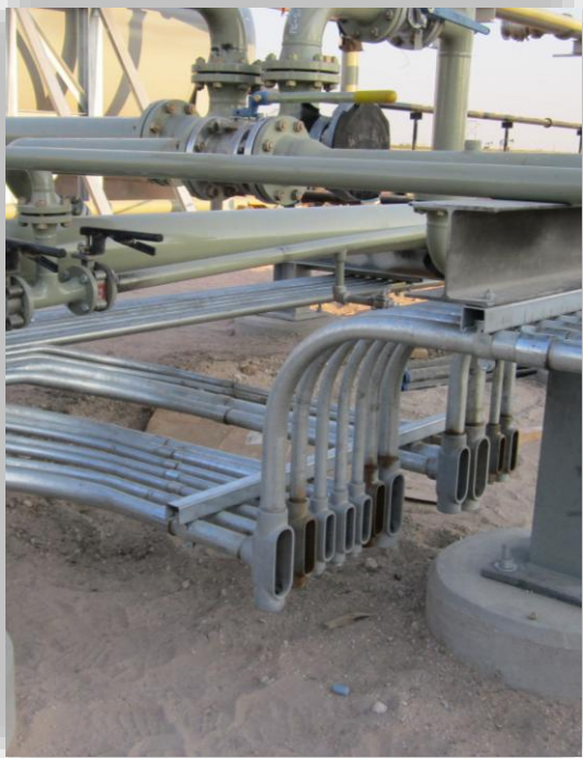
Gas Plant in Texas
